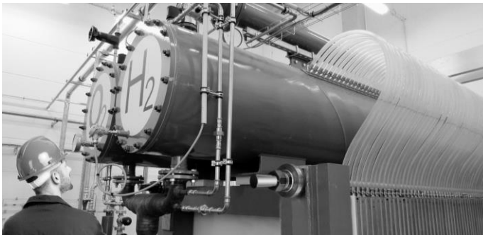
Electrolyser in the past
